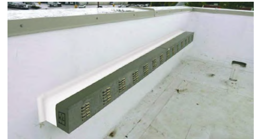
For Reference Only CHS.PP_RW_24LTR RACEWAY FOR 24" LETTERSET INSTALLED BEHIND THE PARAPET SCALE: NTS
